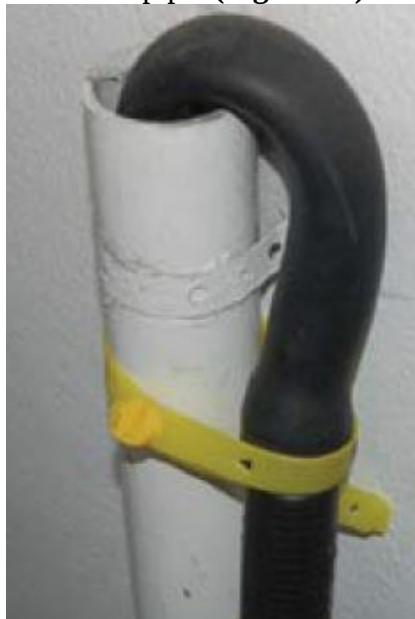
Figure 15. Washing machine drain hose.
